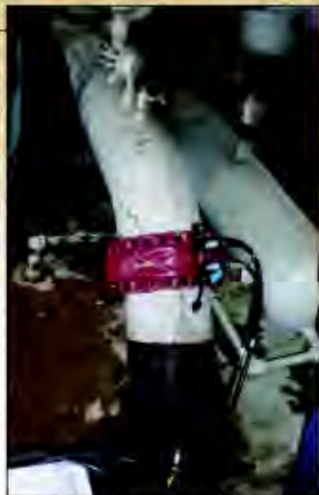
FIGURE 3. Direct methods such as guided wave ultrasonics can inspect lengths of piping from a single test point.
