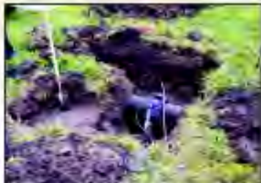
FIGURE 1 and 2. The primary cost of evaluating buried piping is attributed to the time spent on preparing excavations to access questionable piping
